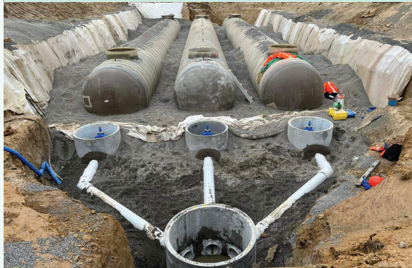
Sanson Wastewater Station
