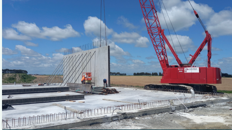
Stanway-Halcombe Water Reservoir
